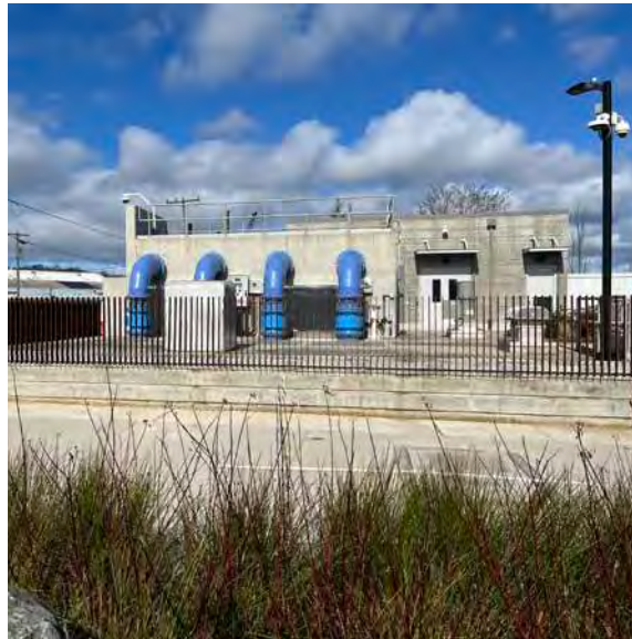
The South Park Pump Station is an example of a grey infrastructure project that provides multiple benefits
